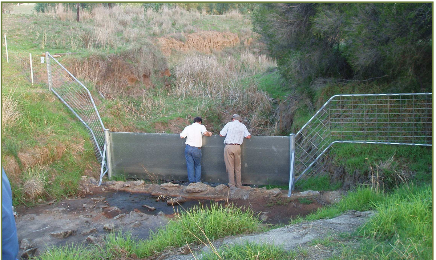
Figure 2: Stabilisation works and flood gates installed with funding obtained through Landcare along Bretton road in Splitters creek
